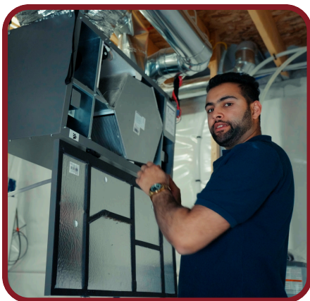
Check every filter in your heating and ventilation equipment.
